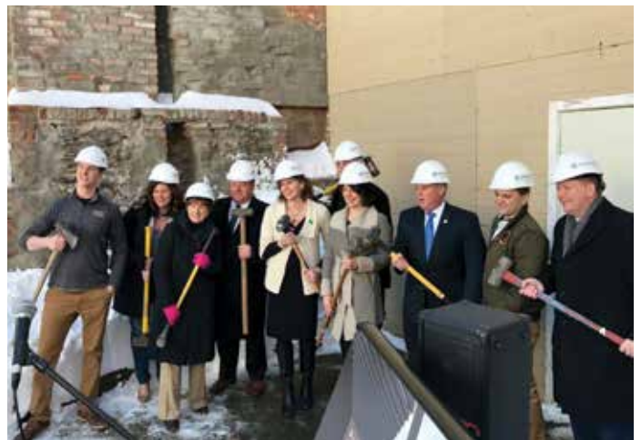
Assemblymember Fahy attends the groundbreaking for the new location of the Albany Distilling Company. Craft brewing and beverages are New York industries experiencing exponential growth in Upstate.
