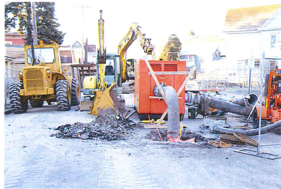
Butternut Street sewer collapse March 24, 2014
